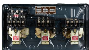
Interior View of MK1 SASD
