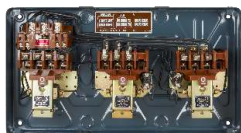
Interior View of MK2 SASD
